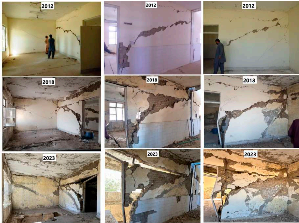
Figure 13. Time sequence photos of progressive damage due to fissure growth over time during the period 2012–2018–2023 at a hospital and adjacent school in the Quetta region.
