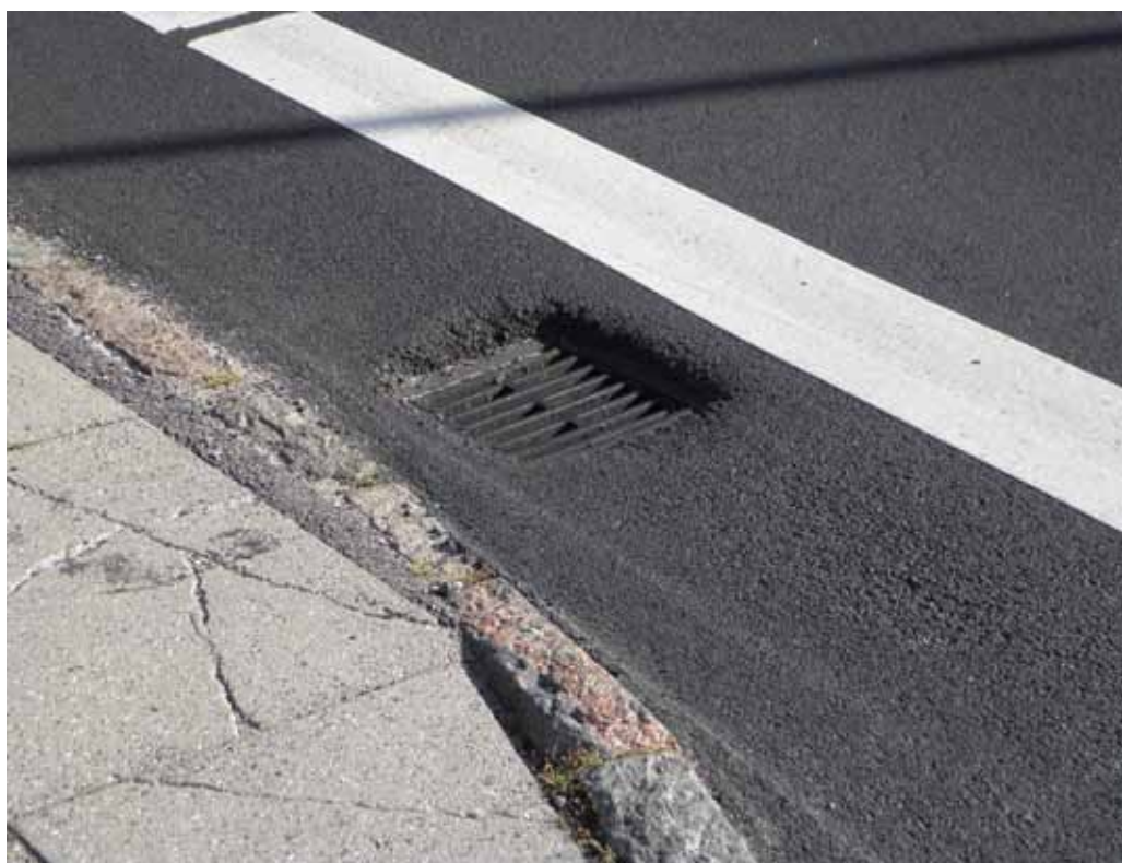
A cycle lane isn't worth much with this kind of gully.
