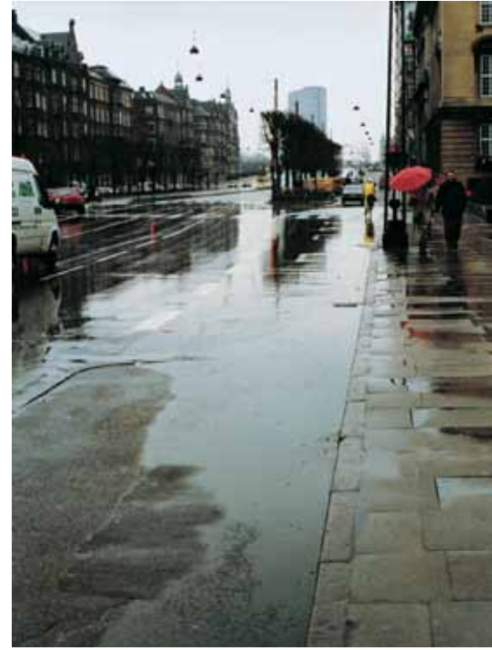
Large puddles make it necessary for cyclists to engage in dangerous dodging manoeuvres.
